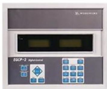
EXISTING EGCP-2 CONTROL
